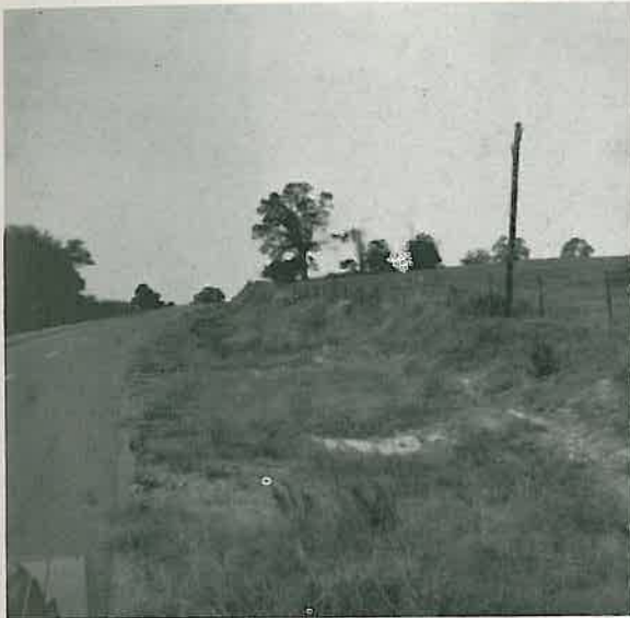
Wide ditch with "Pre-mix" ditch checks one year after construction. On State Highway 53, one mile south of Bodcaw.
