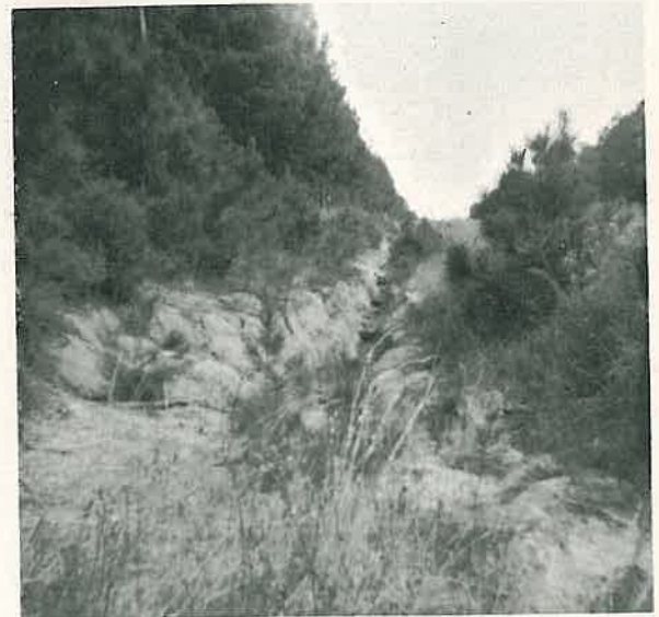
Side ditch erosion. S.H. 53, two miles north of Bodcaw.
